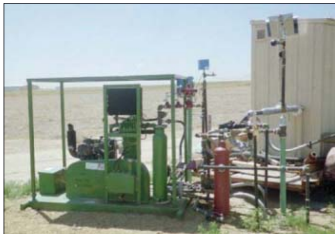
Noble has more than 100 of these packaged two-stage reciprocating compressor VRUs in service in Weld County operations (Fig. 5).
