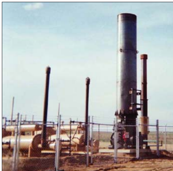
The largest stack in this facility is a 48-in. diameter enclosed flare (Fig. 4).
